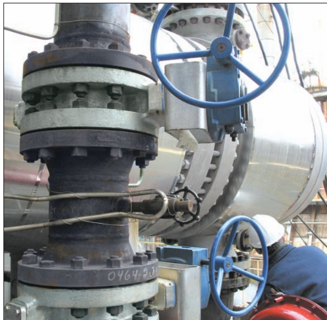
A double block and bleed setup using a 12" (300 mm) class 300 347 stainless steel Torqseal™ valve on hydrogen service at 500 psi/900°F (34.5 bar/482°C).
