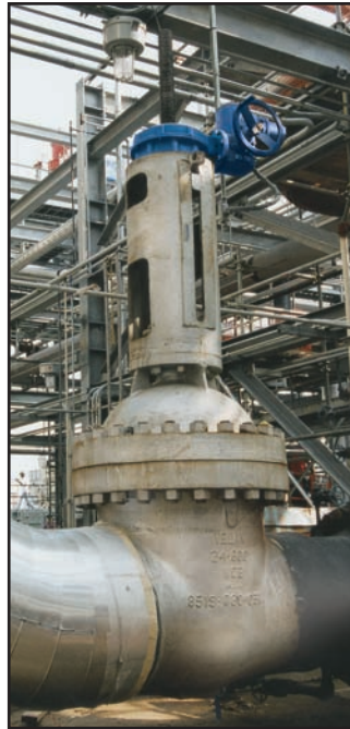
24" (600 mm) cast steel gate valve in hydrocarbon service.
