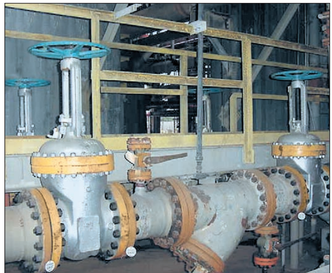
Two HF acid 12" (300 mm) class 300 gate valves installed at ExxonMobil.
