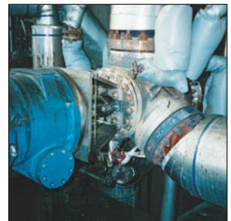
12" (300 mm) switch valve in a delayed coker unit.
