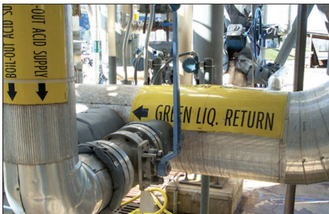
Velan metal-seated ball valves on a new evaporation installation.
