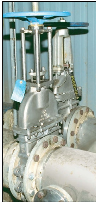
A filter isolation installation of Velan knife gate valves.
