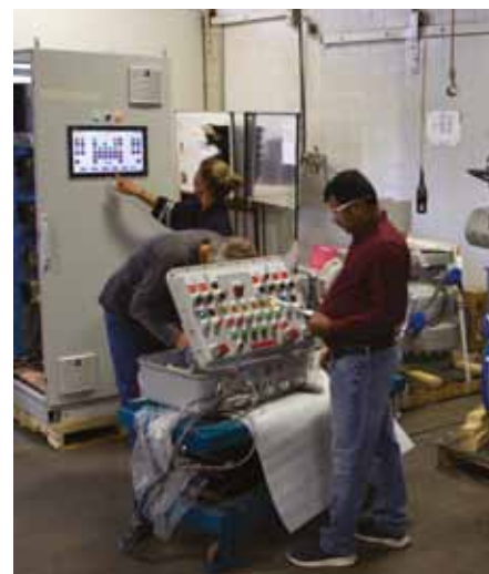
Velan Programmable Logic Controller and control panel
