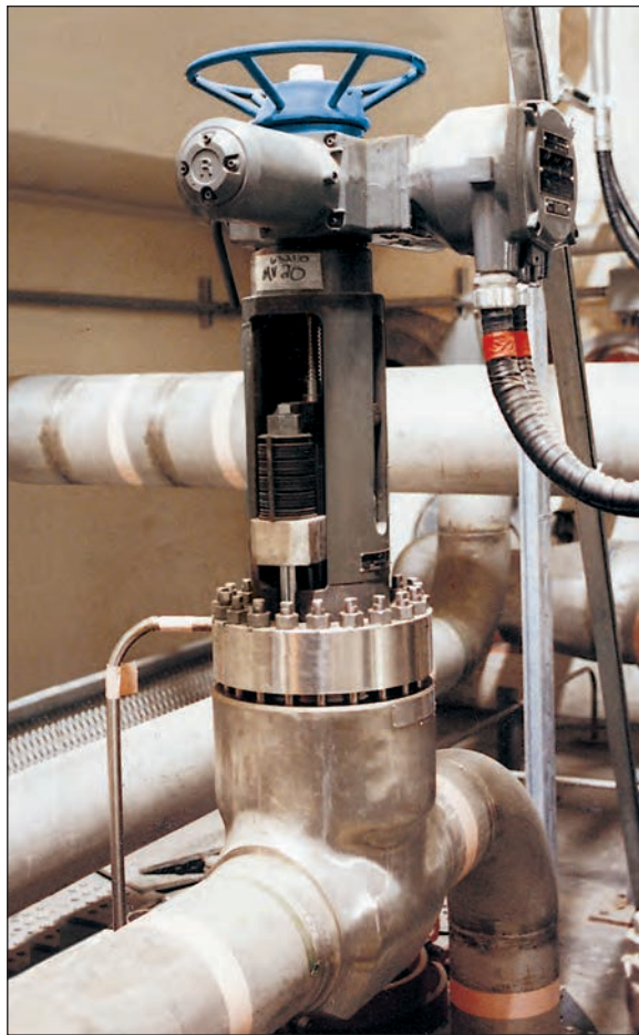
A Velan bolted bonnet valve in a PHT transfer system.
