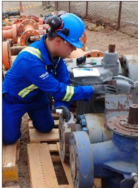
On-site service for Velan valves.
